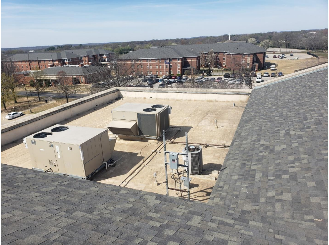
Area 3 – Contractor responsible to remove and reinstall all roof top HVAC equipment, gas, electrical, lightning protection, etc. as required to installed new TPO roofing systems.
