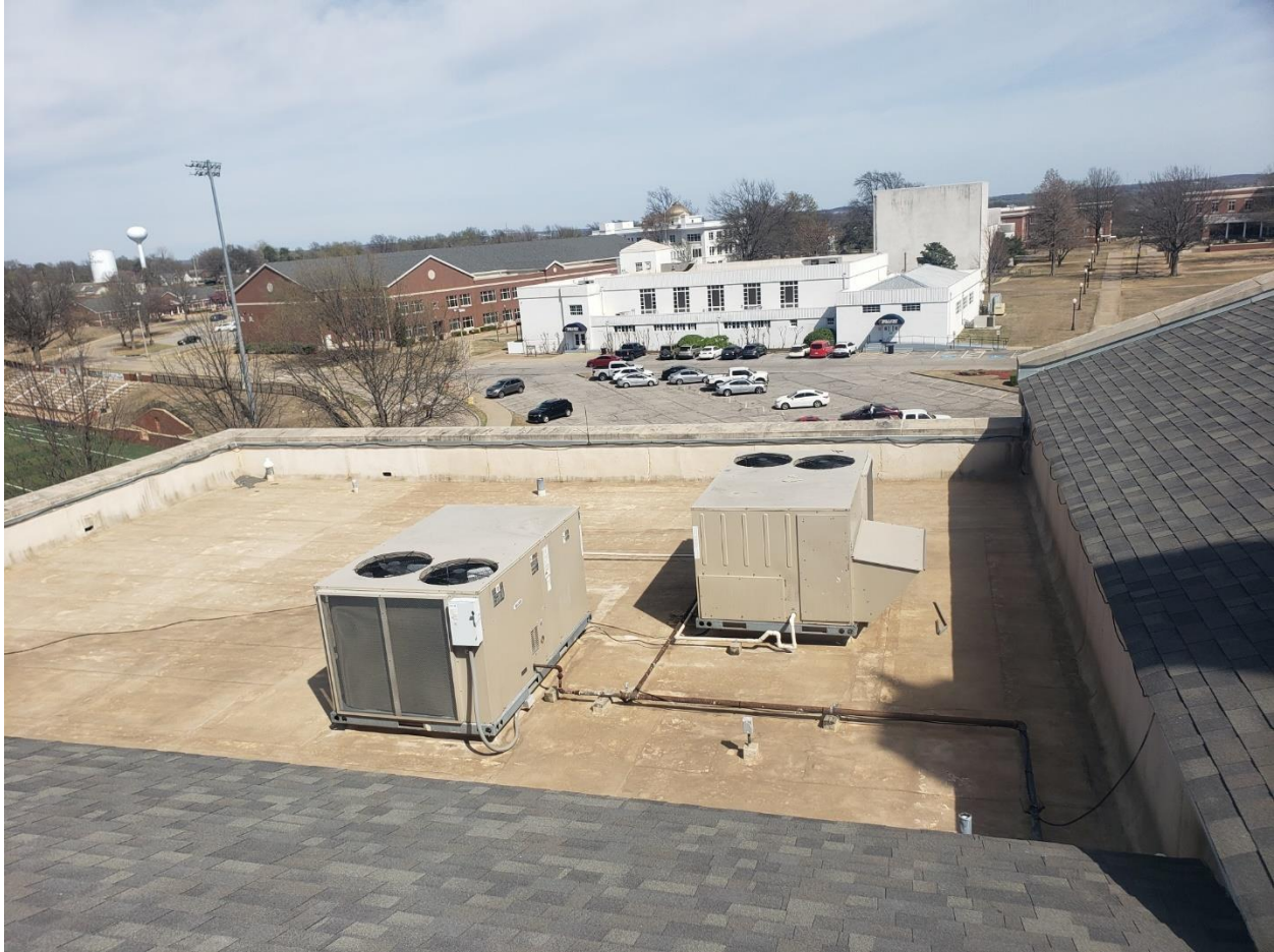
Area 4 – Contractor responsible to remove and reinstall all roof top HVAC equipment, gas, electrical, lightning protection, etc. as required to installed new TPO roofing systems.
