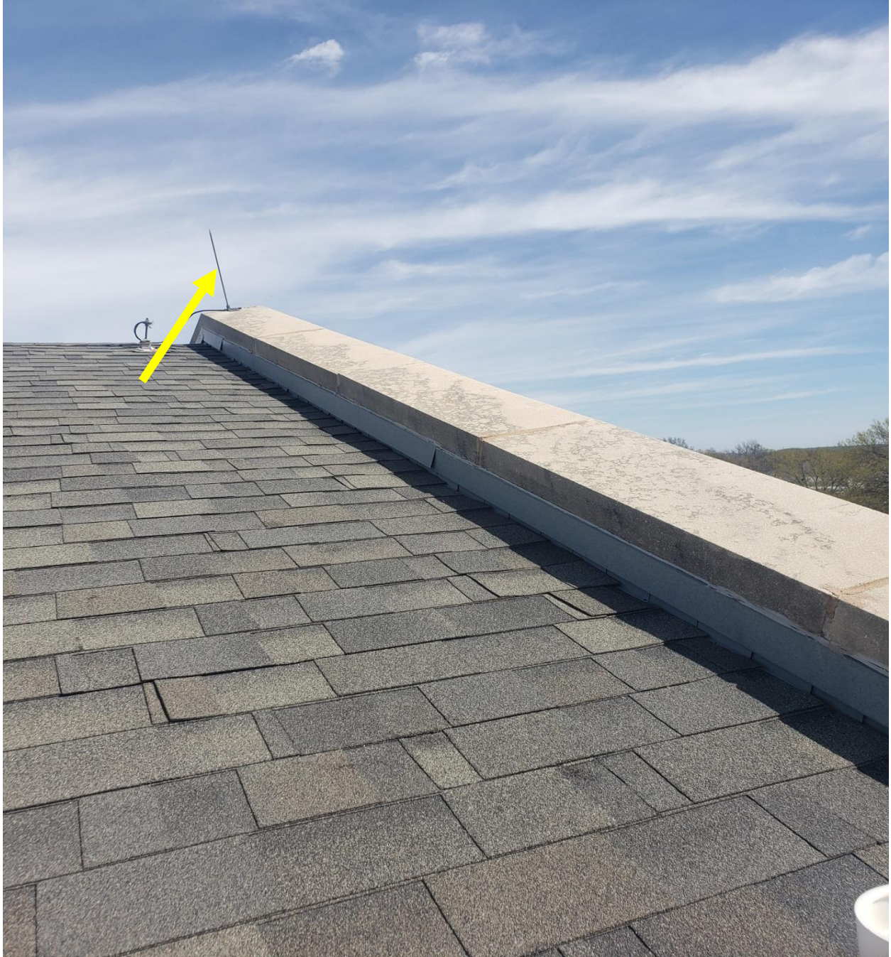
Contractor shall have lightning protection removed and reinstalled by licensed professional.
