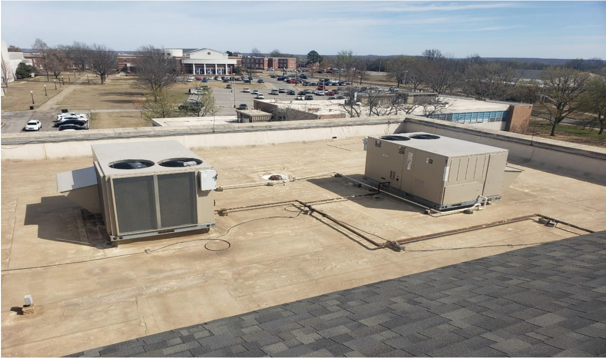
Area 2 – Contractor responsible to remove and reinstall all roof top HVAC equipment, gas, electrical, lightning protection, etc. as required to installed new TPO roofing systems.
