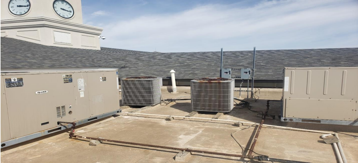
Area 1 – Contractor responsible to remove and reinstall all roof top HVAC equipment, gas, electrical, lightning protection, etc. as required to installed new TPO roofing systems.
